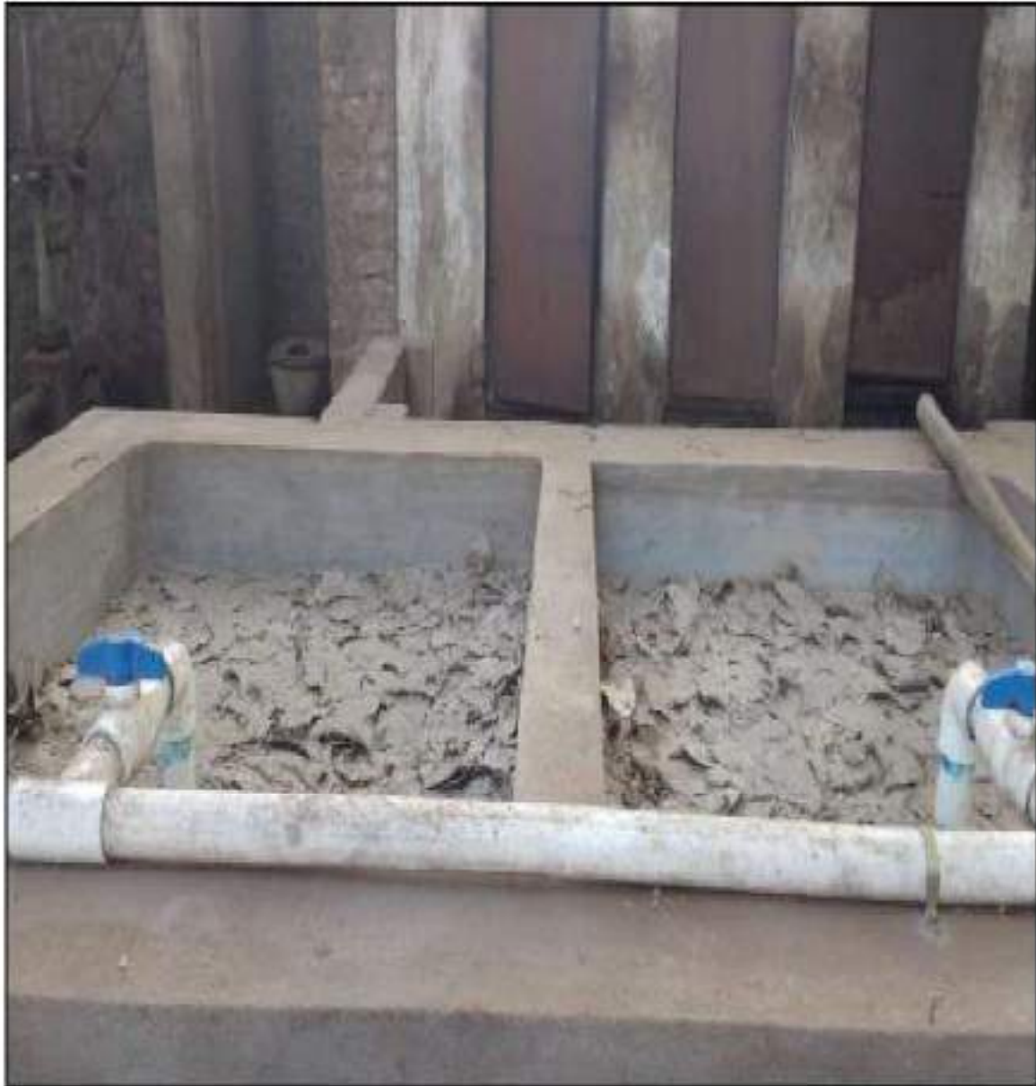
SLUDGE DRYING BED
